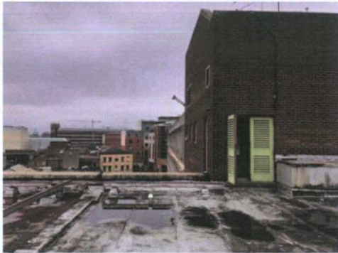
Plate 19: East roof — West 2
