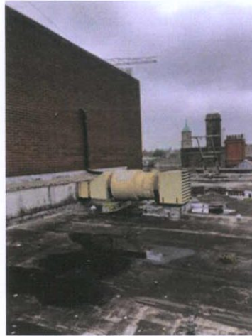
Plate 12: East roof — Ventilation unit
