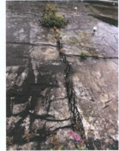
Plate 28: West roof — cracking
