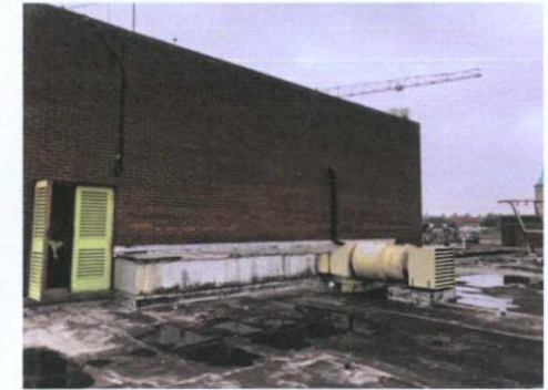
Plate 18: East roof — West 1
