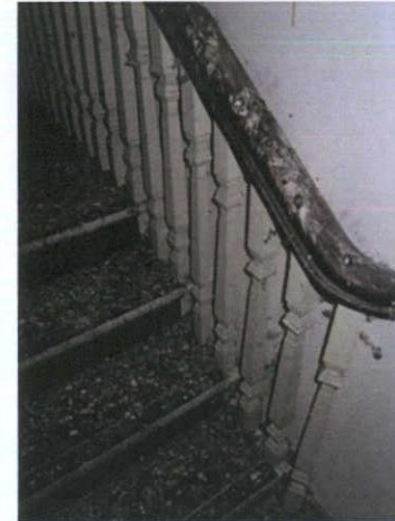
Plate 52: F-4 - Timber balustrade to staircase in main building; first floor staircase cut off from ground floor access
