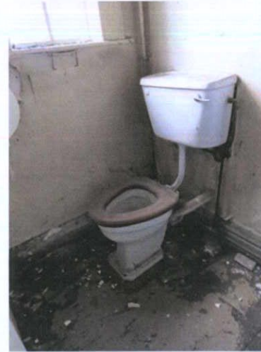
Plate 69: S-2 – Defunct sanitaryware (no photo key on figure 6, p6, S-2)
