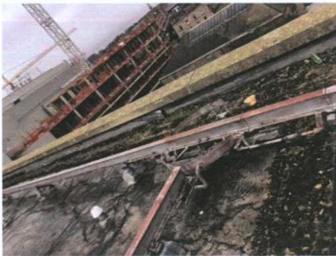
Plate 29: West roof — track for cleaning windows
