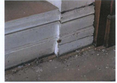
Plate 57: F-5 – Detail to skirting
