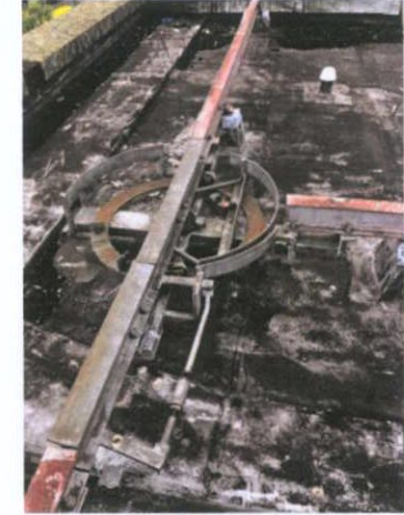
Plate 23: East roof — track for window cleaning crane
