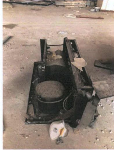
Plate 214: Typical ventilation unit from underneath windows
