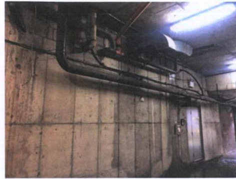
Plate 93: Building services on west wall
