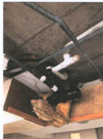
Plate 361: Exposed drainage pipes in ceiling
