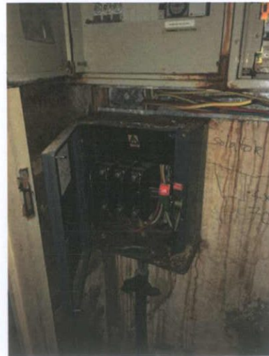
Plate 496: Electrical unit at doorway from west stairwell
