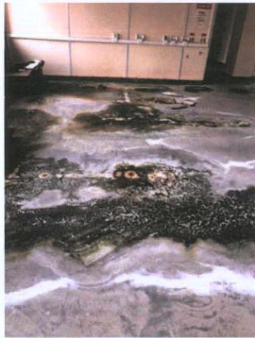
Plate 423: Room 7 — Rot on floor
