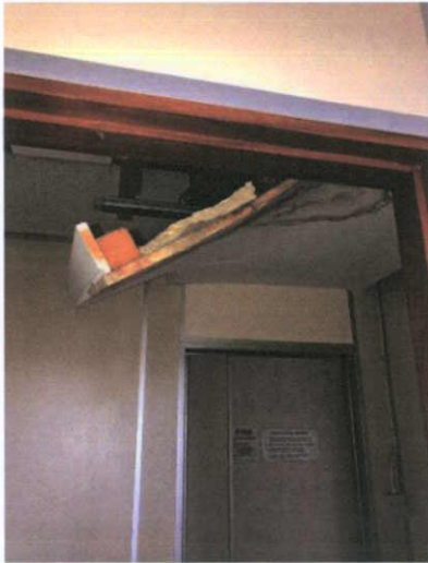
Plate 451: Damage to ceiling in secondary hallway
