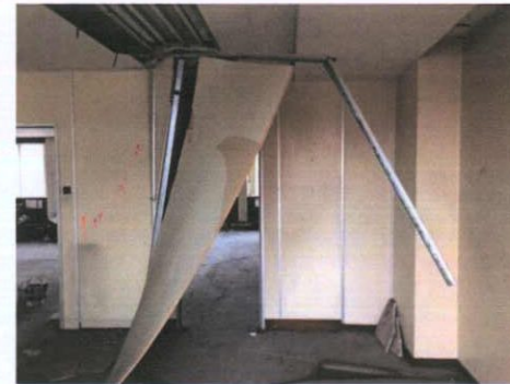
Plate 338: South wall showing damaged partition
