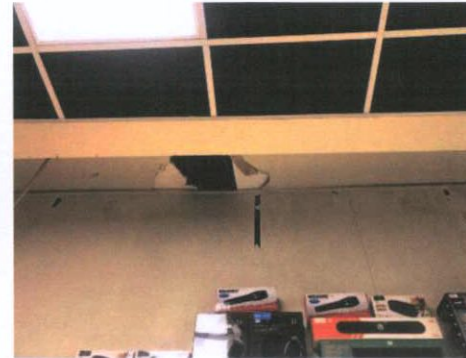
Plate 44: Damage to ceiling in main retail space
