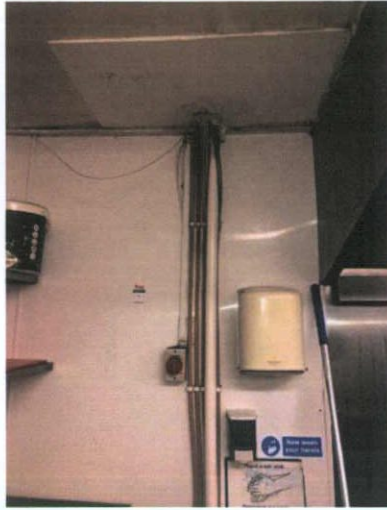
Plate 148: Services entering kitchen
