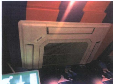
Plate 120: Air Conditioning unit blocked by partition wall
