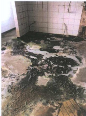
Plate 400: Rot due to leaking roof
