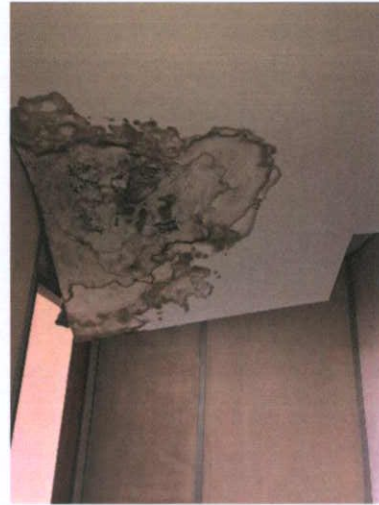
Plate 452: Damage to ceiling in secondary hallway
