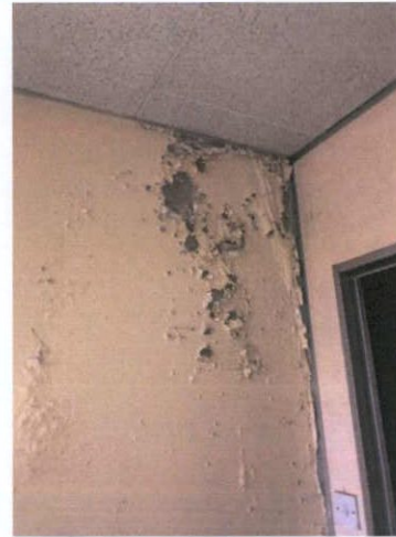
Plate 469: Room 15 — Damage to east wall
