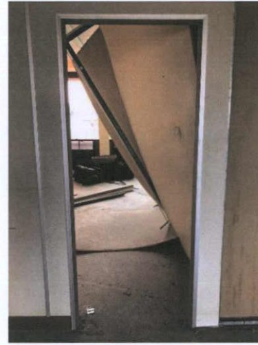
Plate 334: Room 1 — Entrance with damaged stud partition
