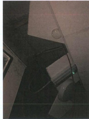
Plate 138: Damage to lighting in fire exit staircase
