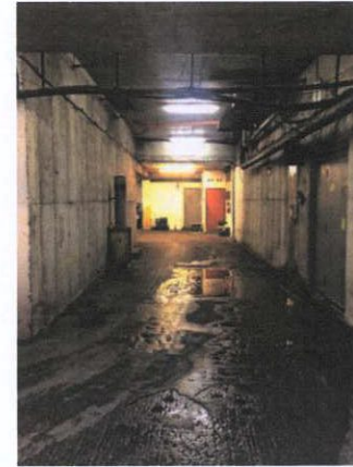
Plate 94: West corridor of car park with retail units fire exits on right
