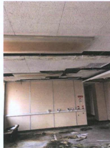
Plate 425: Room 7 — Ceiling damage
