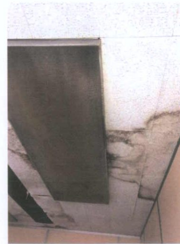
Plate 449: Room 11 — Ceiling water damage
