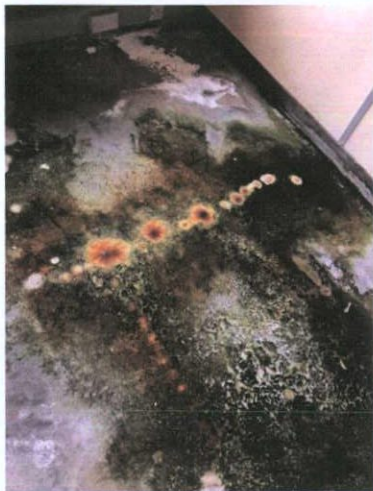
Plate 439: Room 9 — Concrete floor covered in rot
