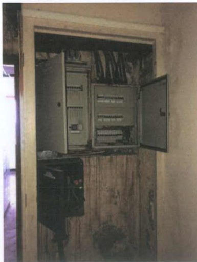
Plate 495: Fuse box at doorway from west stairwell
