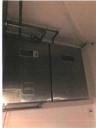
Plate 149: Fire suppression system located in kitchen
