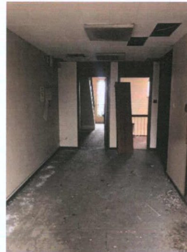
Plate 489: Lift lobby — South wall including east stairwell doorway and hallway to roofs
