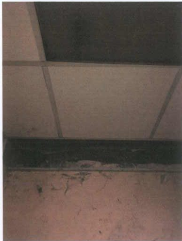
Plate 415: Room 3 — Ceiling damage
