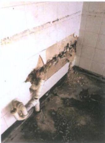
Plate 399: Damage to wall
