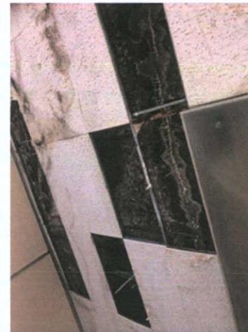
Plate 457: Room 12 — Roof leaking into room
