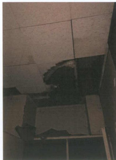
Plate 296: Damage to ceiling of kitchenette
