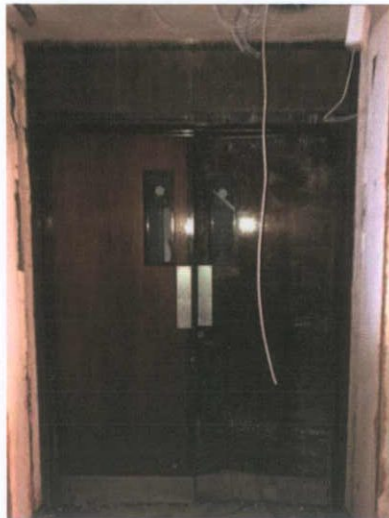
Plate 225: Exit doors to front of building that have been blocked up behind to separate areas
