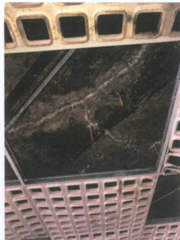
Plate 432: Room 8 — Water leaking through ceiling
