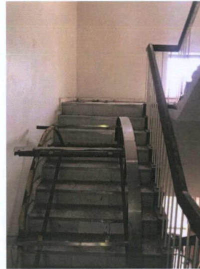
Plate 507: Storage on stair blocking path
