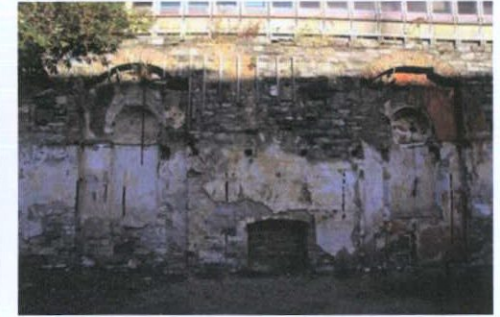
Plate 5: View to north; former chimney breast and flanking niches set into arches; formerly within Number 50
