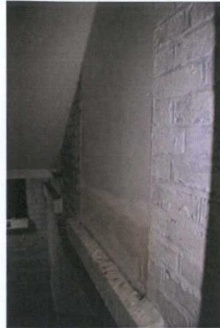
Plate 31: G-1 - Blocked window at side of stairway
