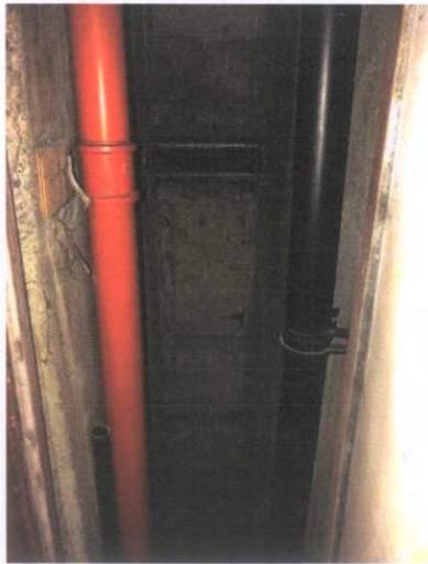
Plate 519: Interior of service riser
