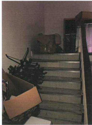
Plate 510: Storage on stair flight
