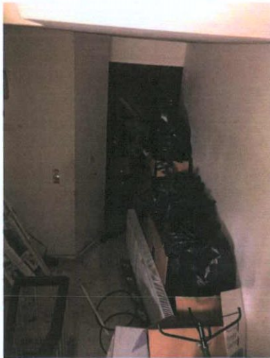
Plate 509: Storage on landing blocking stairs
