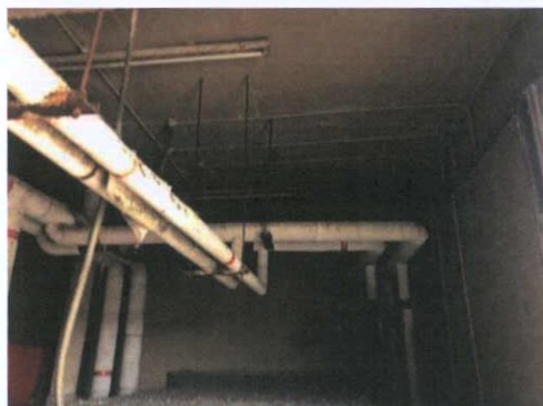
Plate 503: Plant room — Services
