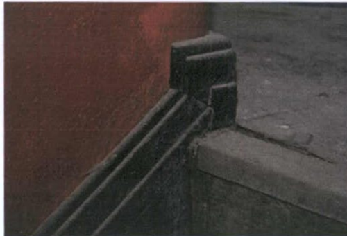
Plate 48: T-5 – Detail to skirting board
