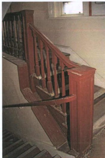
Plate 79: T-1 – View to north-west; original balustrade design resumes from third floor landing to fourth floor
