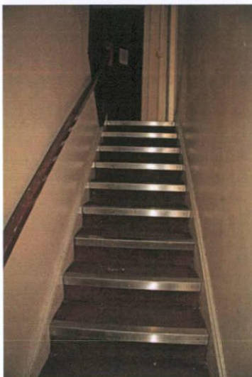
Plate 78: T-1 – View to east; timber stud enclosure to upper flights of stairwell to north (left)
