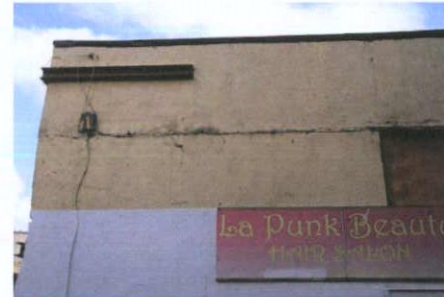
Plate 8: Former slit window, now blocked-up, noted to first floor to south elevation
