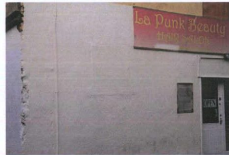
Plate 7: Ghost mark of former window opening
