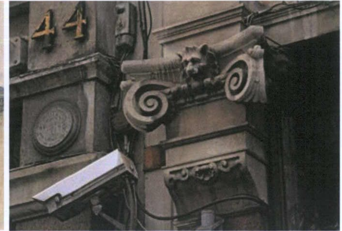
Fig. 10 Carved Portland stone Ionic order capital with lions' head detail. Masonry will be gently cleaned to remove soiling. Redundant services and fixtures to be removed.
