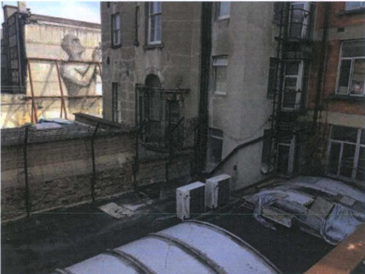
Fig. 4 The eastern end of the boundary wall is attached to the rear of No.42. The flat roof above the rear extension of No.43 is dressed into the boundary wall.
