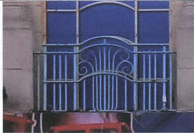
Fig. 31 Decorative railings at first floor level between bays, to be restored and refinished.
