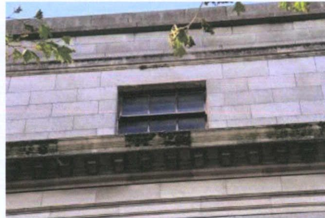
Fig. 27 Dentilled granite cornice at third floor level to be inspected at close range and lead flashing applied if required.
