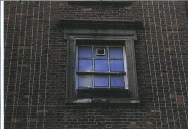
Fig. 58 Level 2 Windows: Moulded Roman cement architraves; granite sills with later rendered finish coat applied, and now failing. The architraves will be retained and repaired.
