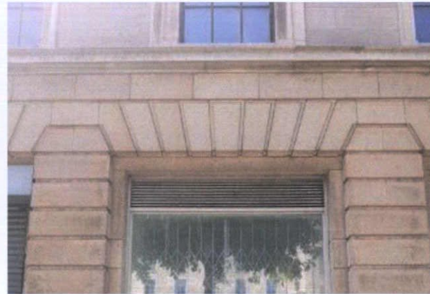
Fig. 24 Square-headed window openings; Late 20 th century windows with ventilation grilles over to be replaced.
