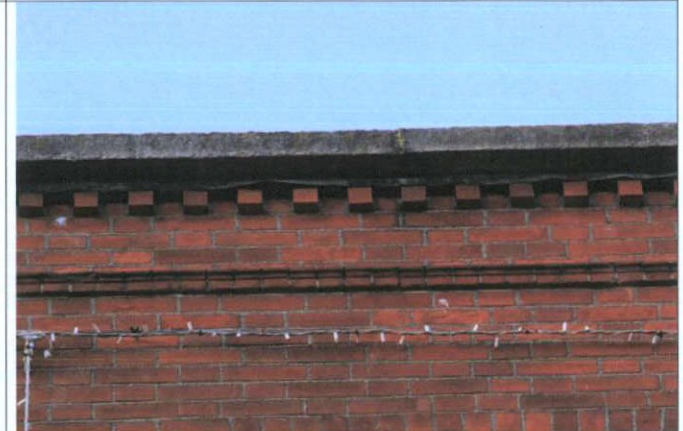
Fig. 60 Detail of the reconstructed parapet, with granite coping on flashing and dentil brick cornice. The brickwork and granite coping will be repointed.
