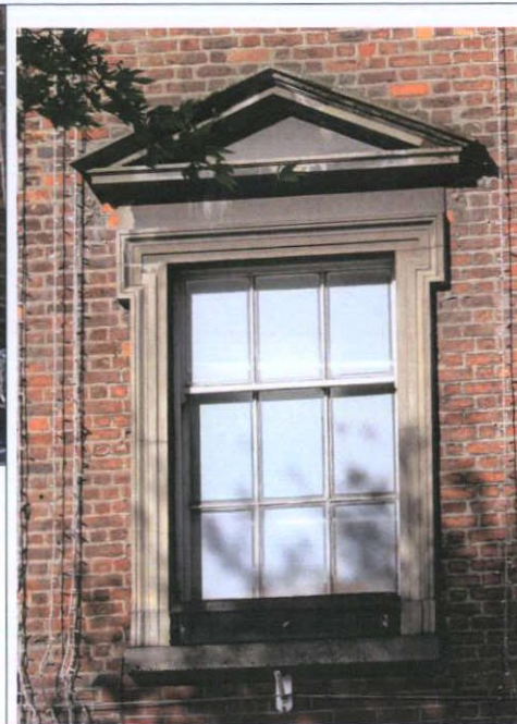
Fig. 57 Level 1 windows: Lugged, Roman cement architraves and hood mouldings, repaired with cement, pedimented to first floor. The architraves will be retained and repaired.
