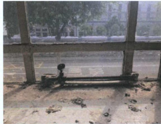
Fig. 19 Detail of metal casement openings, original fixings intact. Steel windows to be restored.
