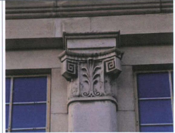
Fig. 33 Detail of art deco inspired detail on capitals. All masonry elements to be gently cleaned to remove graffiti and soiling.
