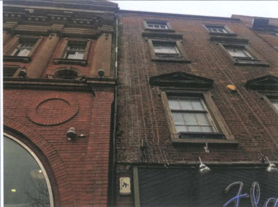
Fig. 61 Detail of eroded pointing and decayed brick behind the rainwater downpipe. The rainwater downpipe will be repaired and replaced to match original profile. Biocide will be applied and vegetation removed. The affected brickwork will require repair and repointing.
