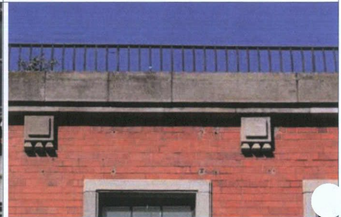
Fig. 44 Parapet railing, damage to brickwork from removed fixings
