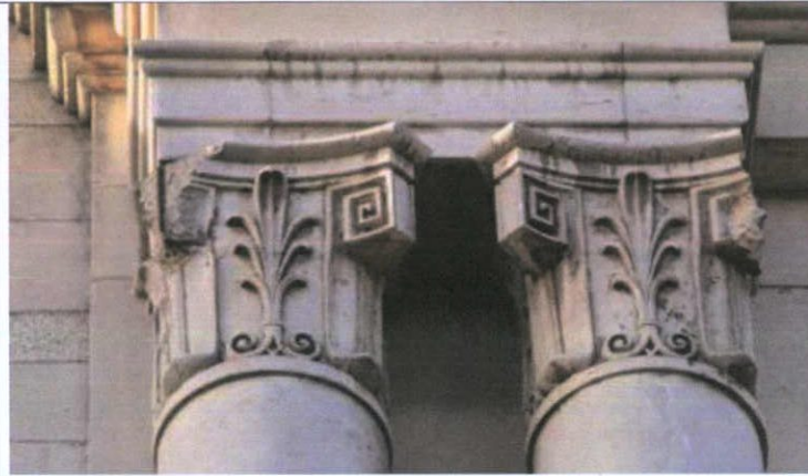
Fig. 35 Example of damage to capitals requiring stone graft repair.
