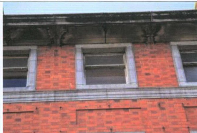
Fig. 51 Granite cornice, with water-staining evident.
