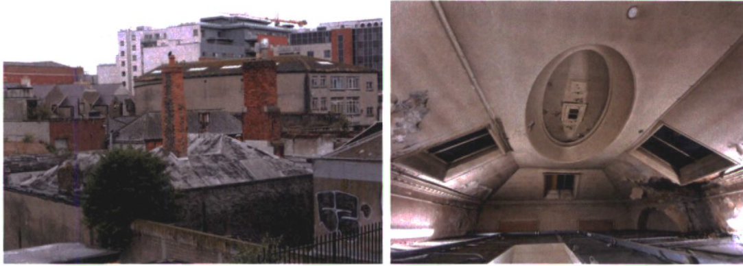
Plate 15.3.10 Roof and interior of rear of a former reading room pertaining to the Sackville Street Club
