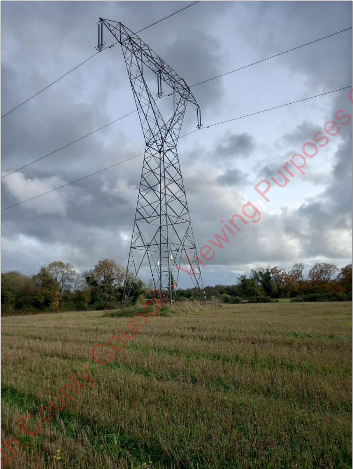
Plate 19.6. View of electricity pylon, facing southwest
