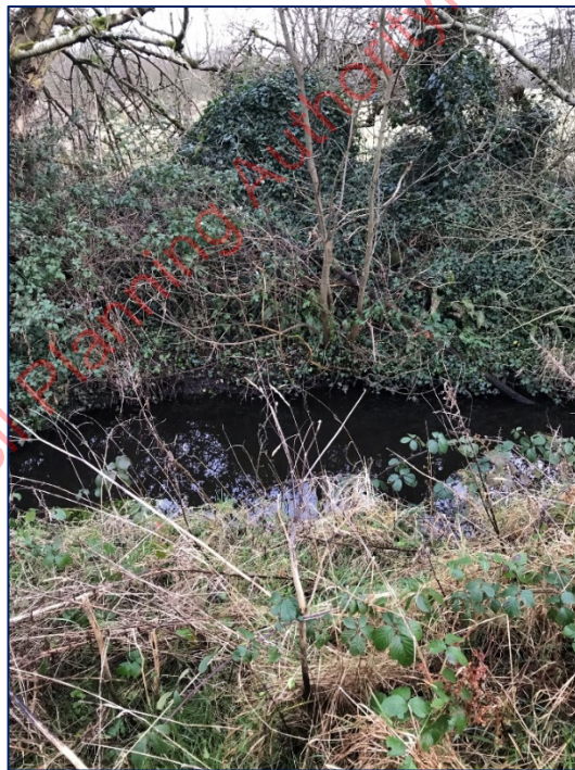
Figure Error! No text of specified style in document.-21: FW2 – Eroding/ Lowland River at the north of the Site (Garrynafela stream)
