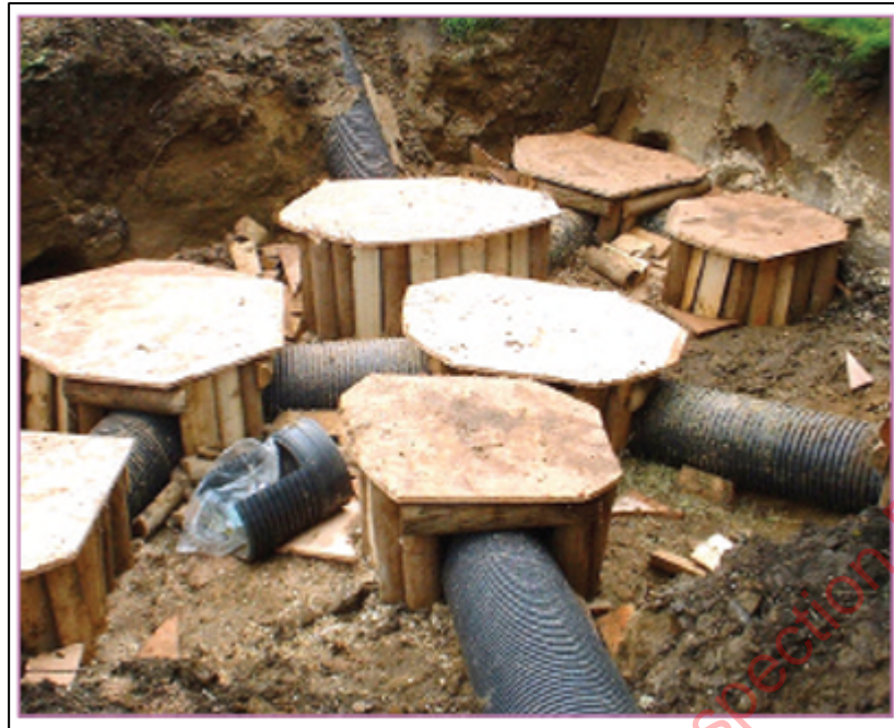
Figure Error! No text of specified style in document.-32: An example of an artificial sett under construction with pipe tunnels and 7 chambers (Extracted from NRA (now TII), 2005b)
