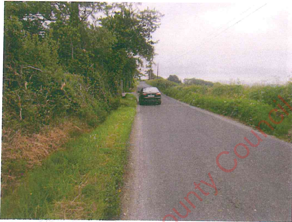
Road Surface at Culvert beside car
