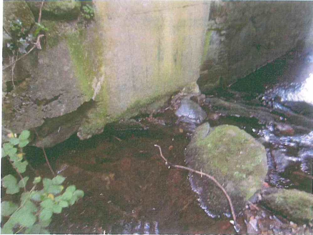
Scouring next Concrete Buttress
