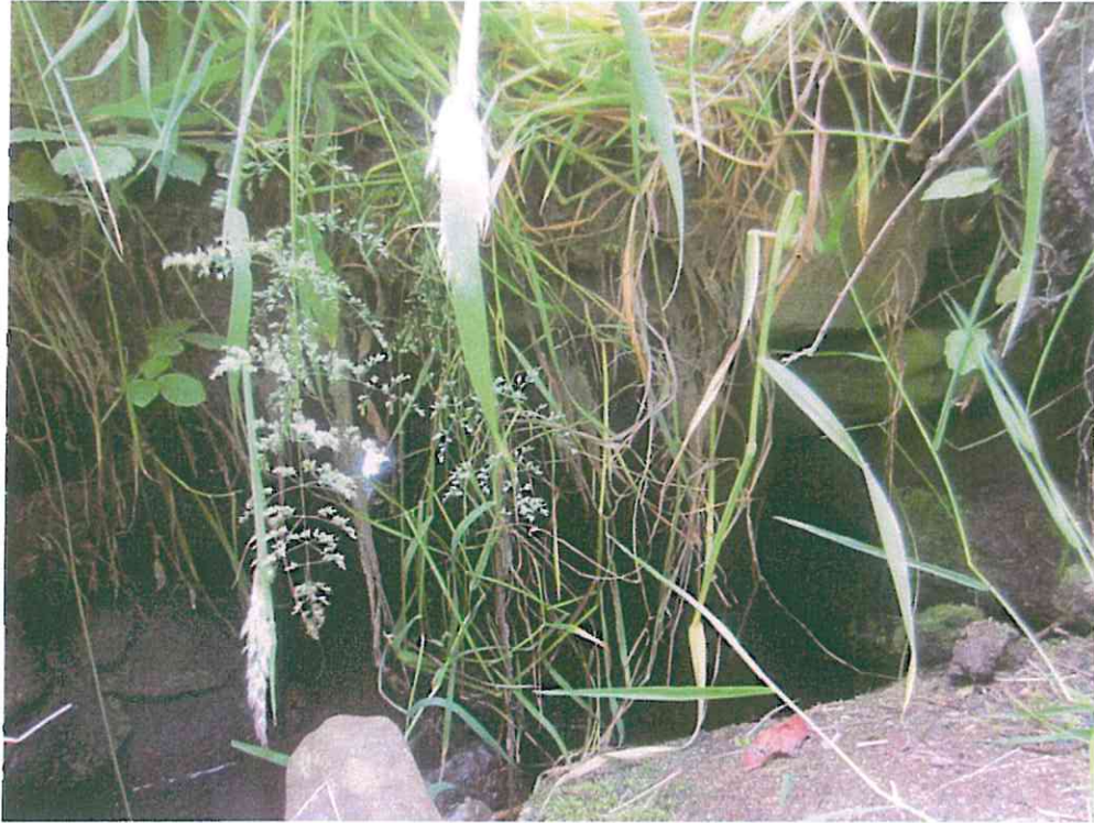
Culvert, 250mm deep arch stone with 350 to finished load level 600mm span
