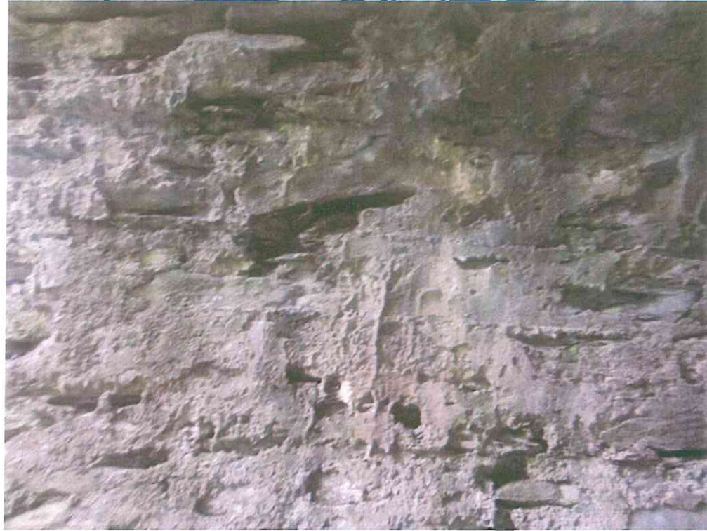
Calcide on Underside of Arch
