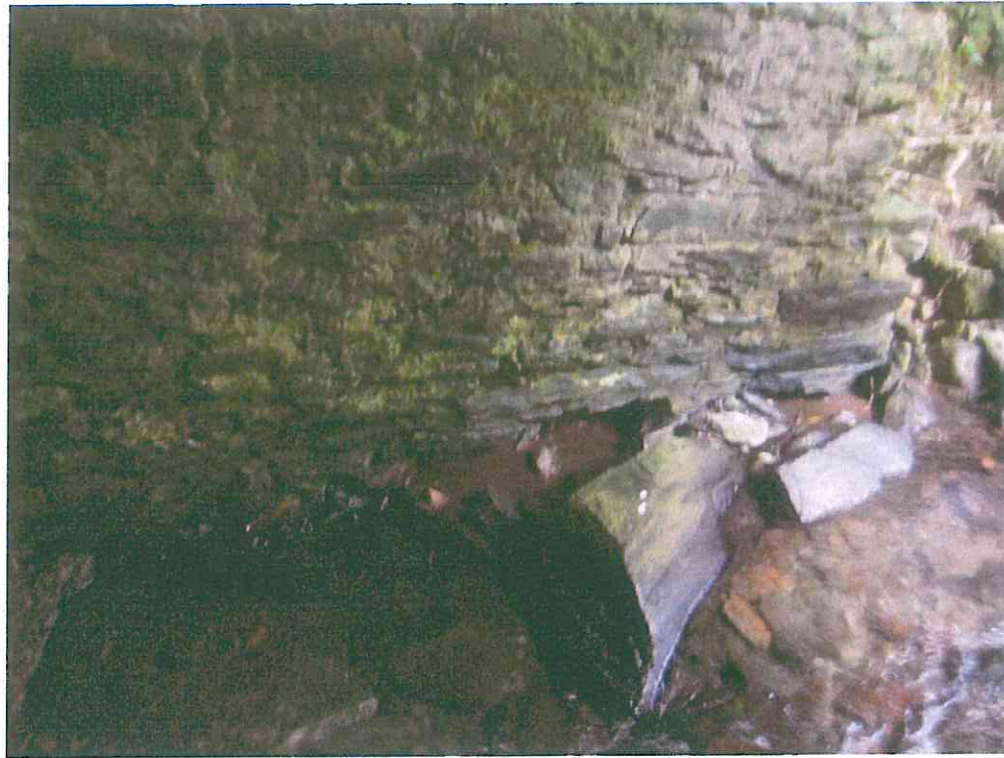
Minor Scouring of Abutment on Upstream Side
