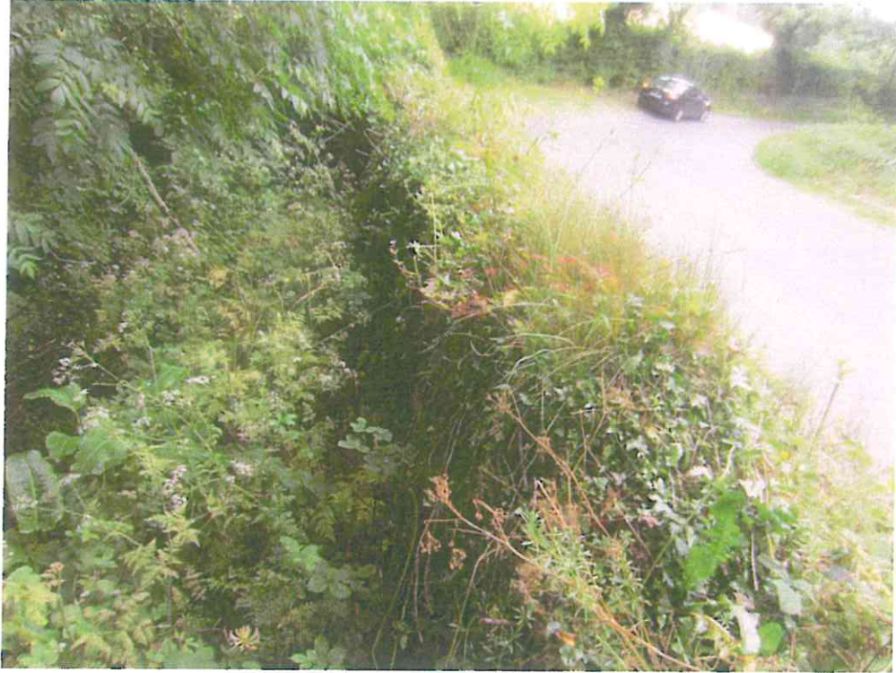
Parapet Wall Overgrown with Ivy-Upstream Side
