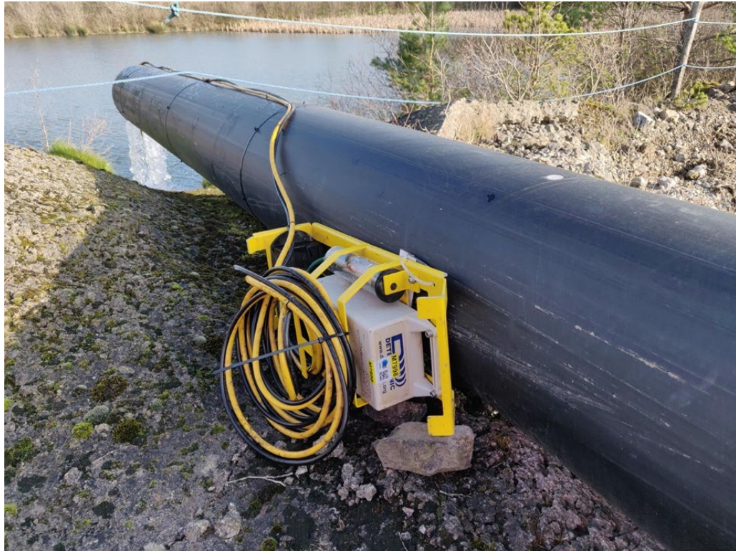
Plate 8.2: CWSL Installation Ultrasonic flowmeter fitted to balancing pond inlet
