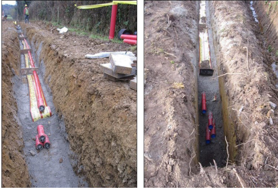
Plate 4-9 Typical Cable Trench View
