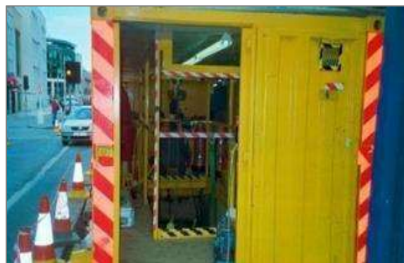
Figure 19: HV Cable Jointing Container
