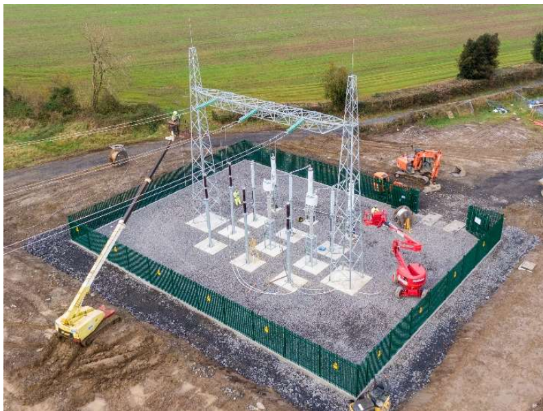
Figure 6 Cable Compound Complete with Gantry
