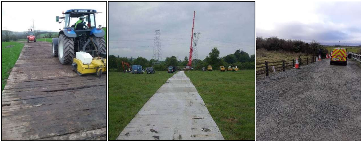
Figure 21: Timber Roadway Bog Matt (Left) Temporary Aluminium Panel Tracks (Middle) Crushed Rock (Right)
