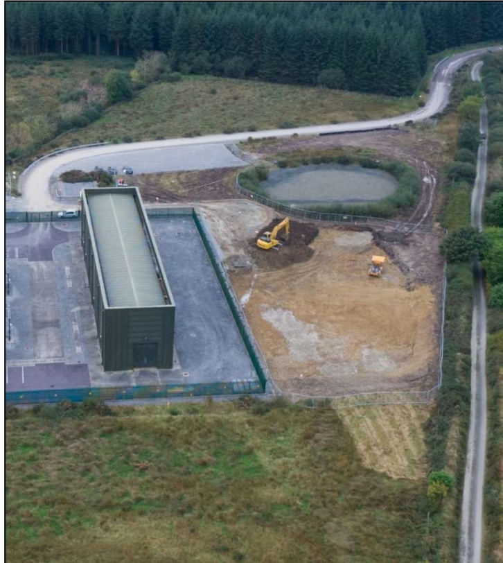
Figure 20: Typical 220kV GIS Switching Substation
