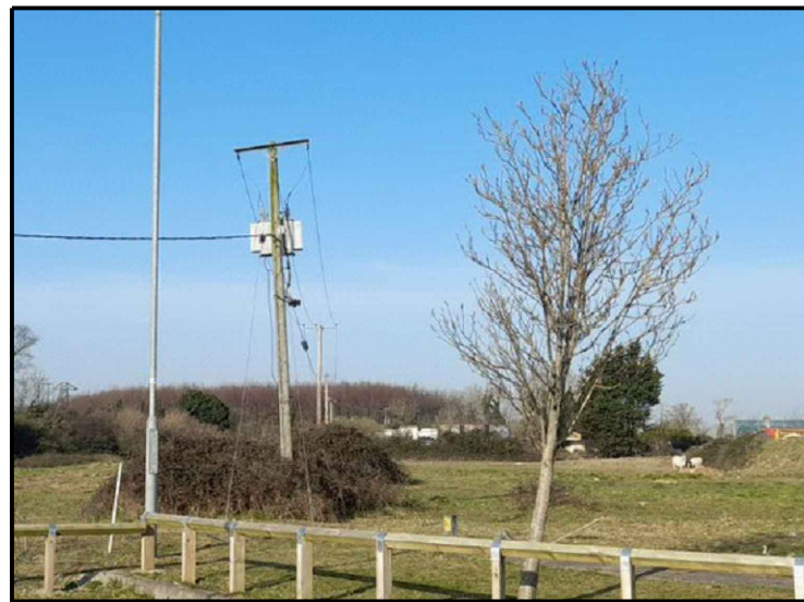
Power Lines to be Decommissioned
