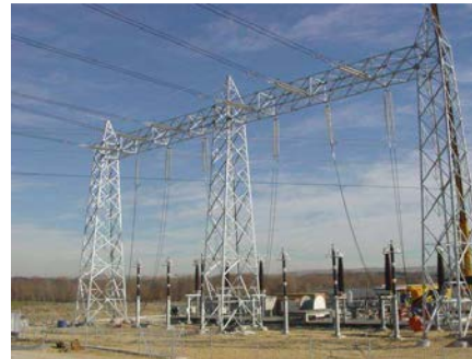
Figure 5: Overhead line cables transition station (400kV)
