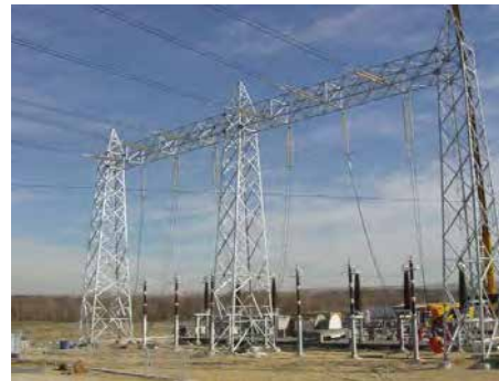
Figure 5: Overhead line cables transition station (400kV)
