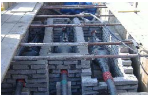
Figure 5.3: Image of 400kV Joint Bay
