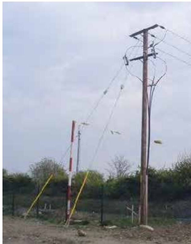
Figure 3-1: A typical MV line/cable interface pole
