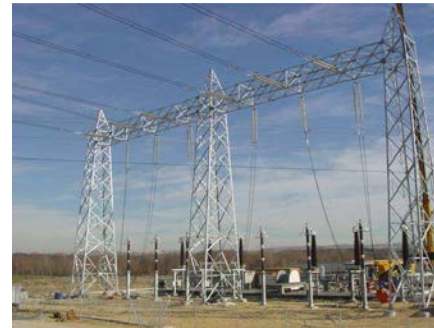
Figure 5: Overhead line cables transition station (400kV)
