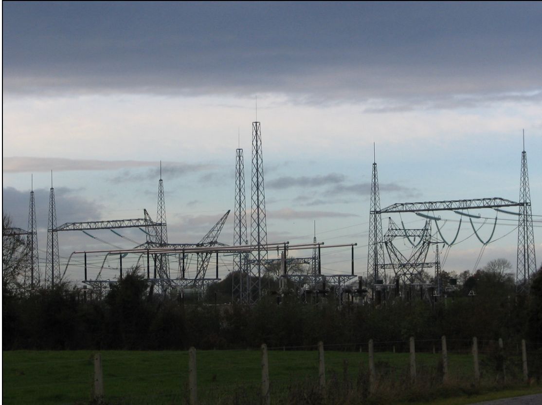
Figure 3.3 Oldstreet 400kV Station
