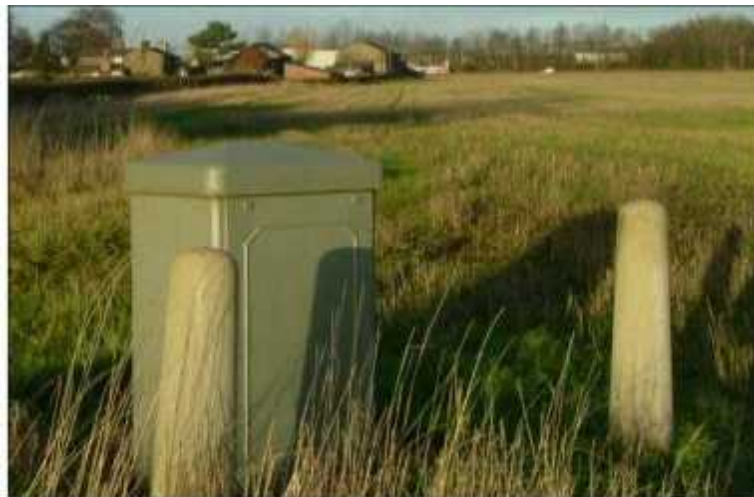
Plate 10.10: Photograph of Above Ground Inspection Kiosks for UGC
