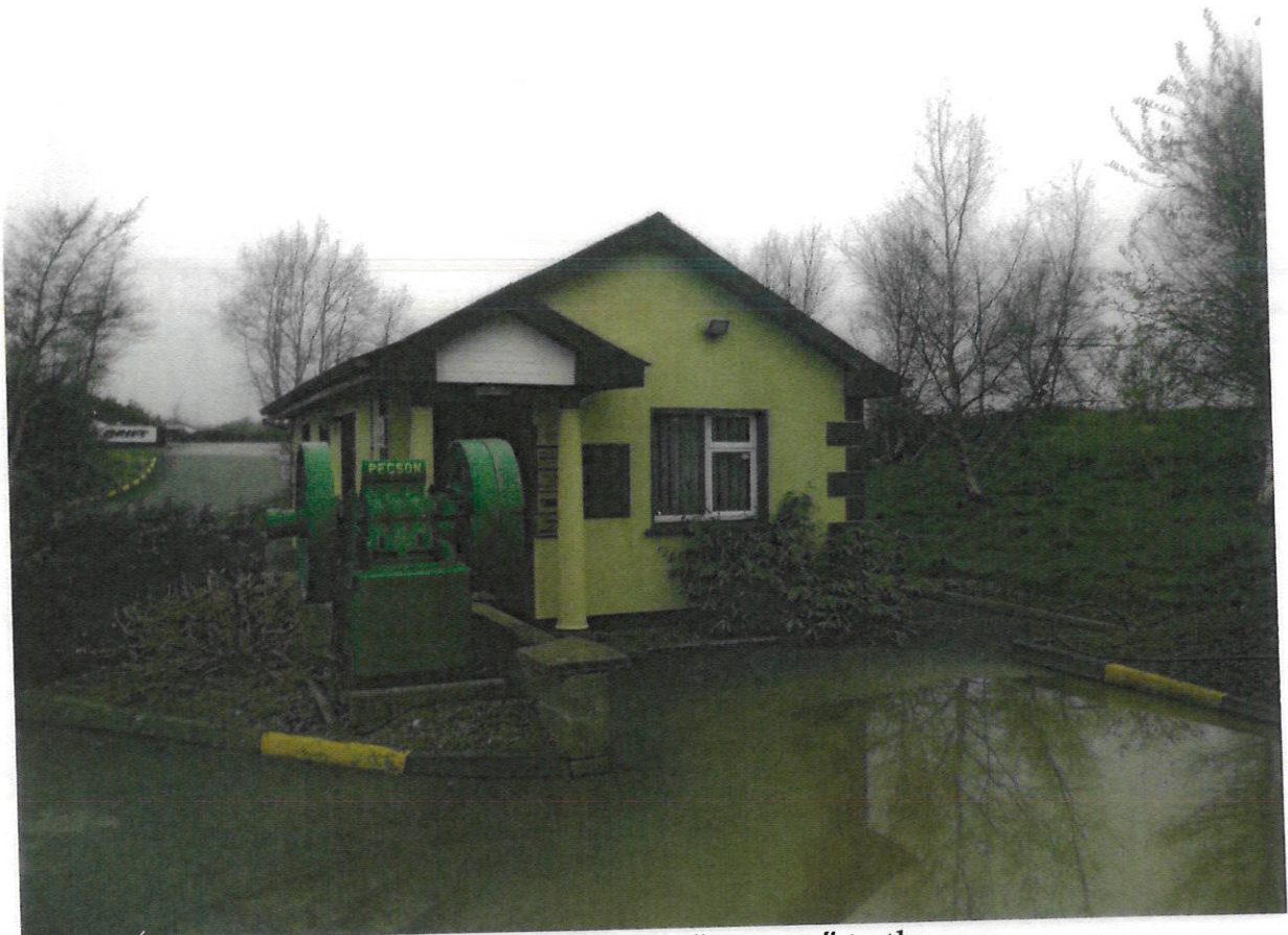
Existing structure used as gents toilet/ office "Pit area" to the rear
