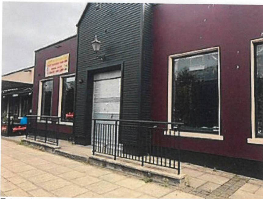
External west façade of the building with the mock up not visible
