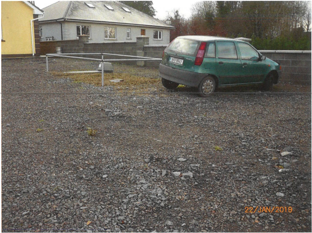
Photo No 2 Percolation area filled over
