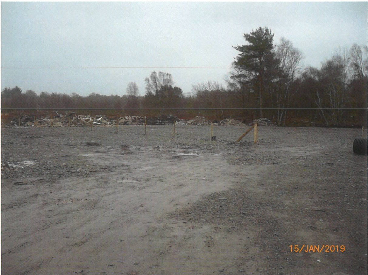
Photo No 12 – Unauthorised Clearance, Drainage, Importation of Construction & Demolition Waste and Filling in Bog Area
