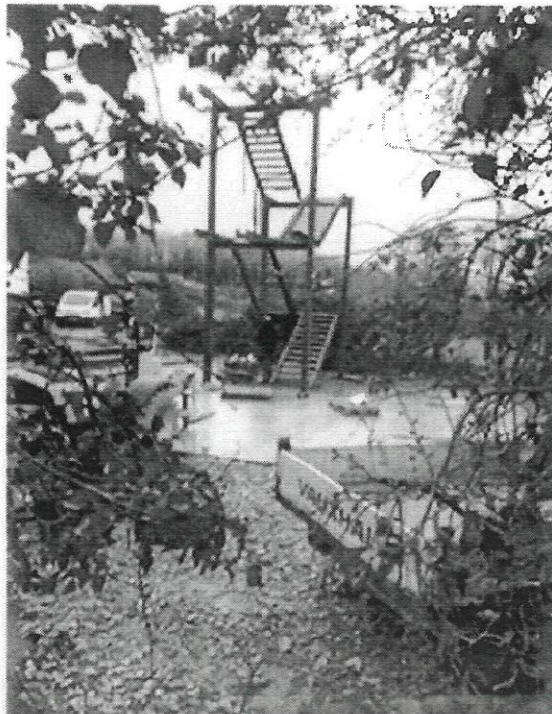
Fabrication of parts of a building occurring in an area shown in 05/1008 as a car park and percolation area for a waste water treatment system.
