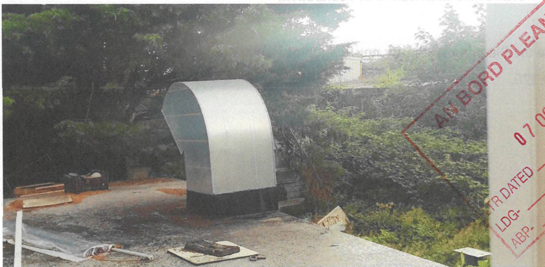
Photograph of Extraction Hood Currently in Place
