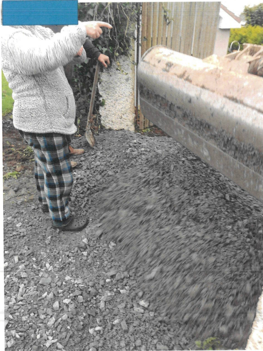
30 June 2020 19:03. Excavator with bucket in motion dropping gravel load dangerously close to concerned neighbour as one of the Excavator crew looks on. No construction safety signage, safety cones or tape.
