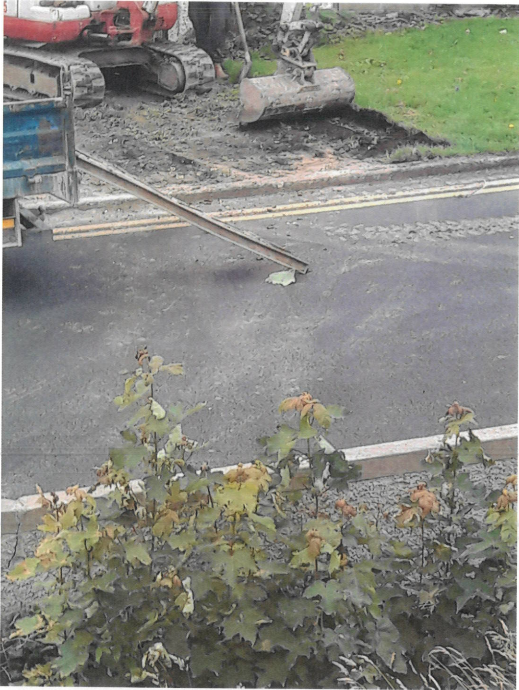
30 th June 2020 18:52. Excavator digging up public green area along blue line markings.
