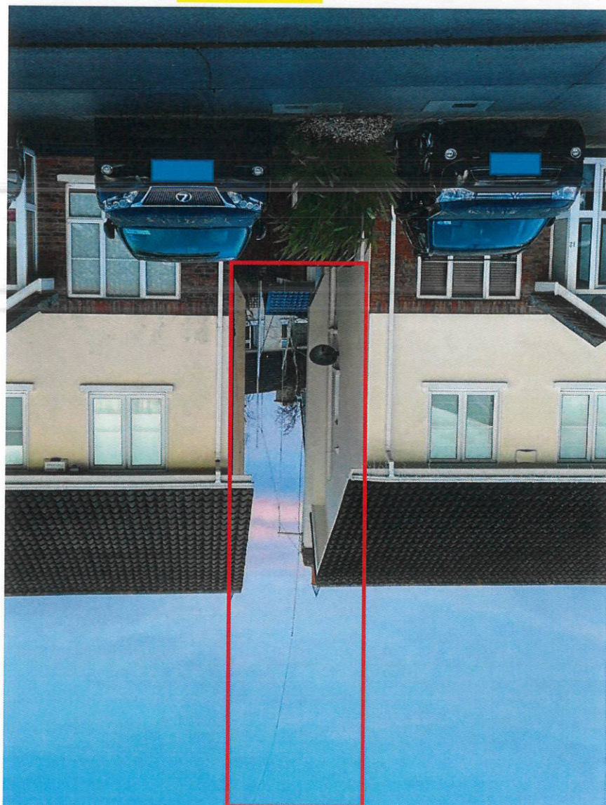
Photo No. 8: This photos taken on 3 rd February 2021 shows the gable elevation to No. 12 (on the left hand side) with the antenna extending up from the chimney and the high level wires linking to the unauthorised development at the rear. There is also a television satellite dish on the gable elevation.
