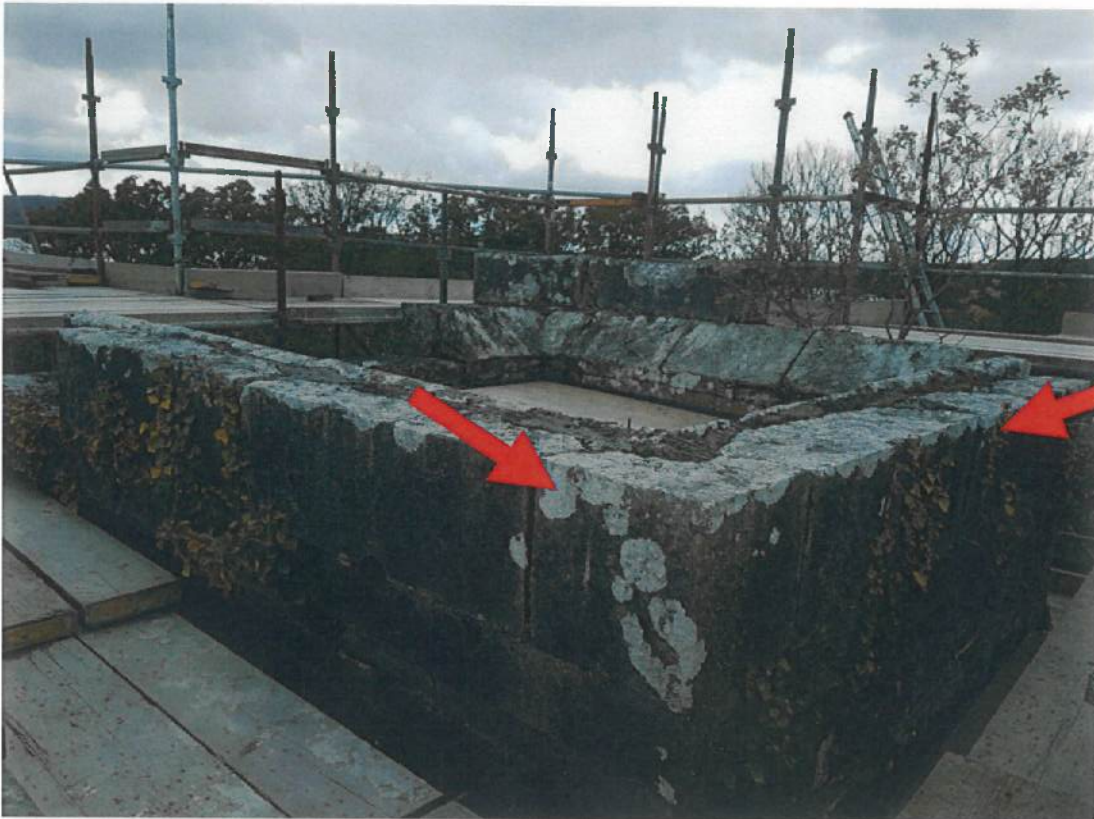
Photograph – taken from high tower – Note poor condition of stonework, including ash tree and loose stones.
