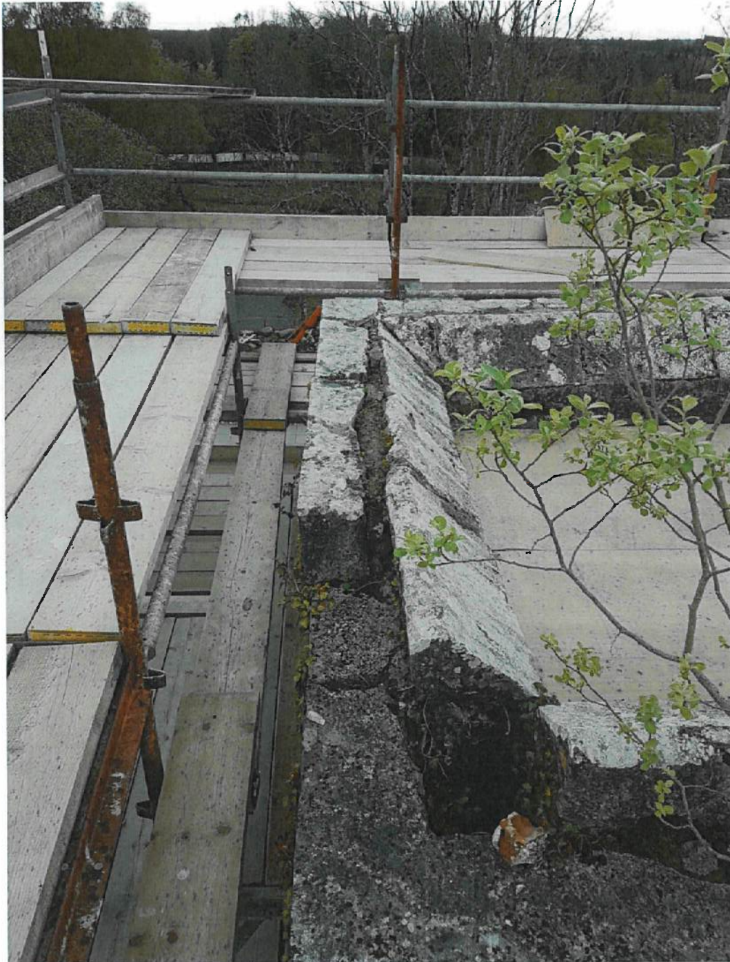
Photograph – taken from high tower – Note poor condition of stonework, including loose stones and gaps developing between inner and outer stones.
