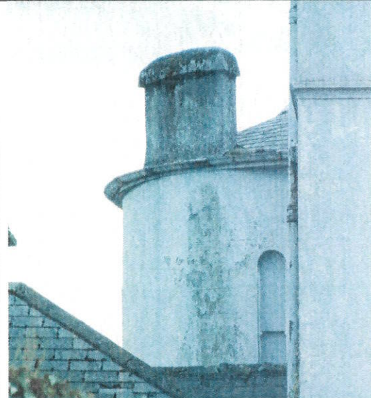
Circular Tower shown on 1565 map of Portlaoise now incorporated into Presentation Convent
