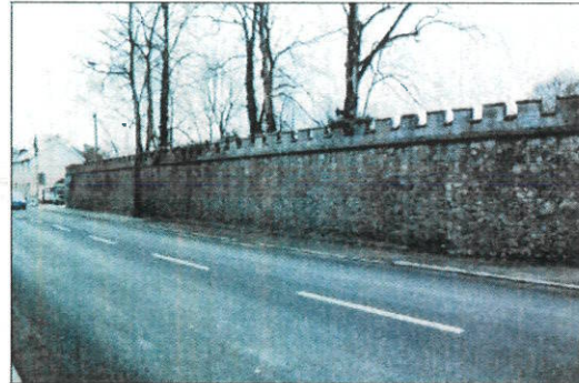
Castle Durrow demesne wall on approach road to south west of village square.
