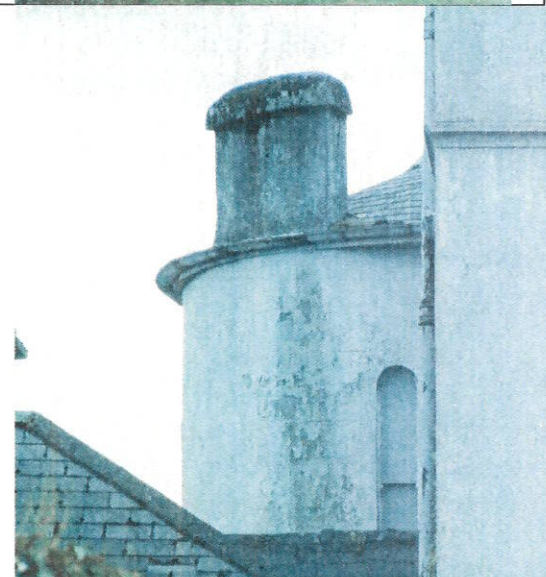
Circular Tower shown on 1565 map of Portlaoise now incorporated into Presentation Convent
