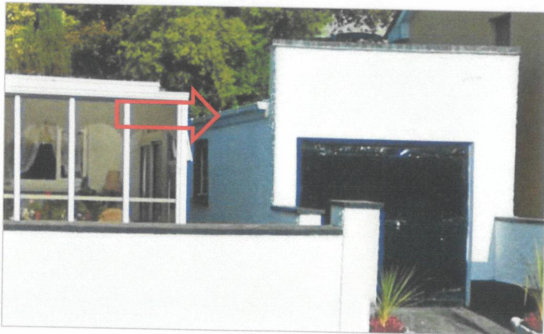
Plate 5 Google earth image of subject site illustrating the previous lower height of monopitch roof on north-western elevation of garage in relation to existing conservatory extension
