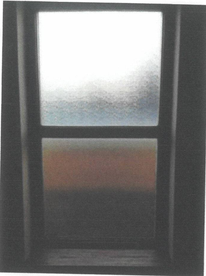
Plate 8 Impact of raised roof on gable window
