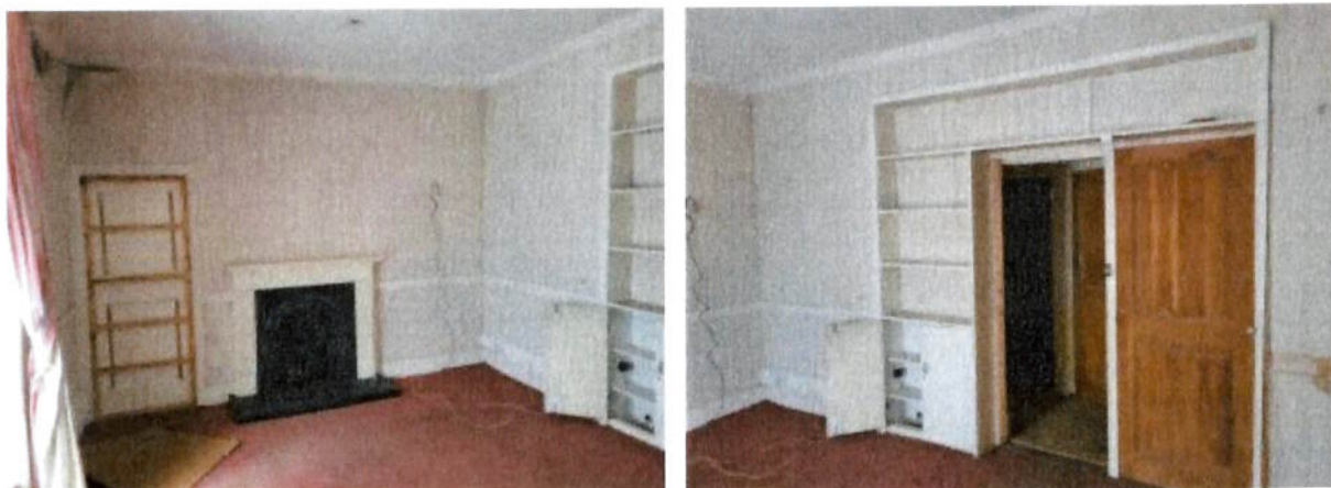
Figure 5.0 A ground-floor bedroom in Hayden's Hotel, as included in the photographic survey carried out on 1 st April 2025.
