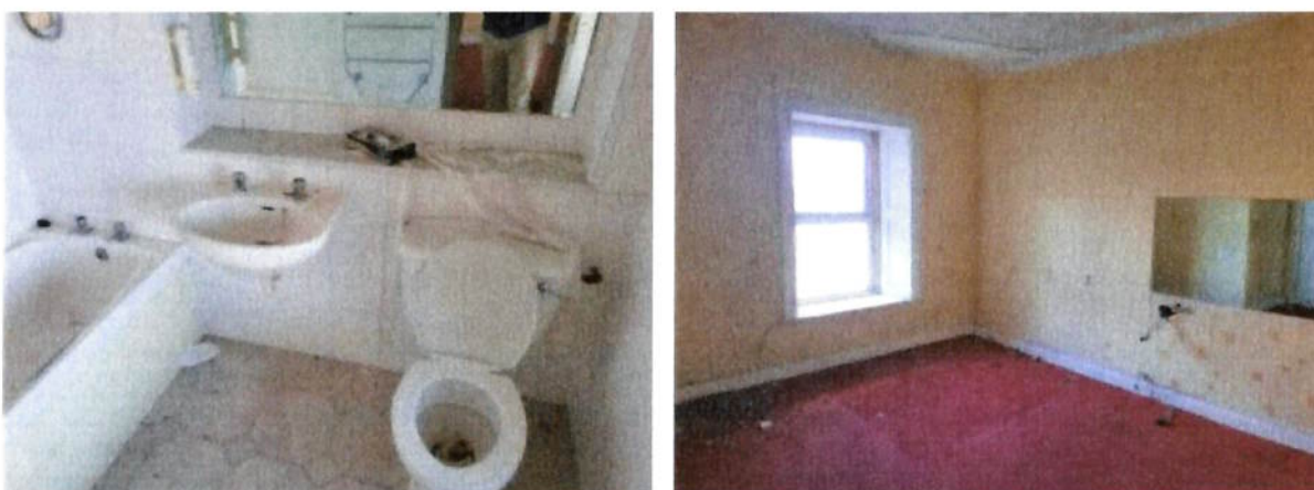
Figure 7.0 A second-floor bedroom and bathroom in Hayden's Hotel, as included in the photographic survey carried out on 1 st April 2025.
